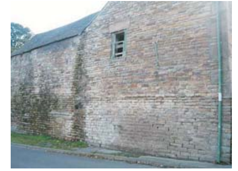
Historic building in need of maintenance.
