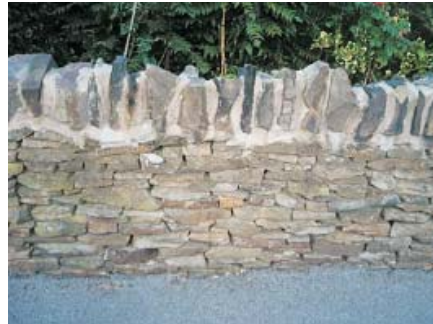
The coping stones of this wall have been repaired with hard cement mortar that has disfigured the appearance of the wall.
