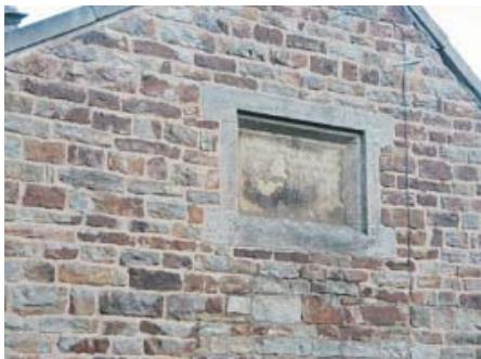
This eroded datestone would benefit from repair.
